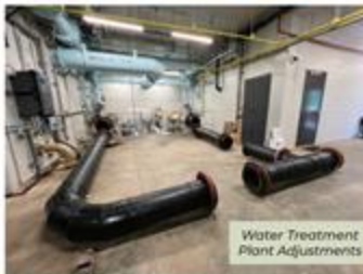
Water Treatment Filter Pilot Project
